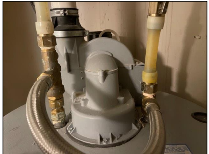
28. PEX connected direct to water heater.
