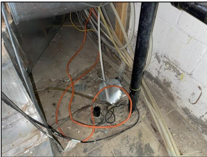
10. Not well secured
