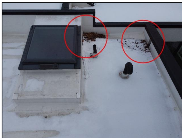
2. Debris/oil on roof
