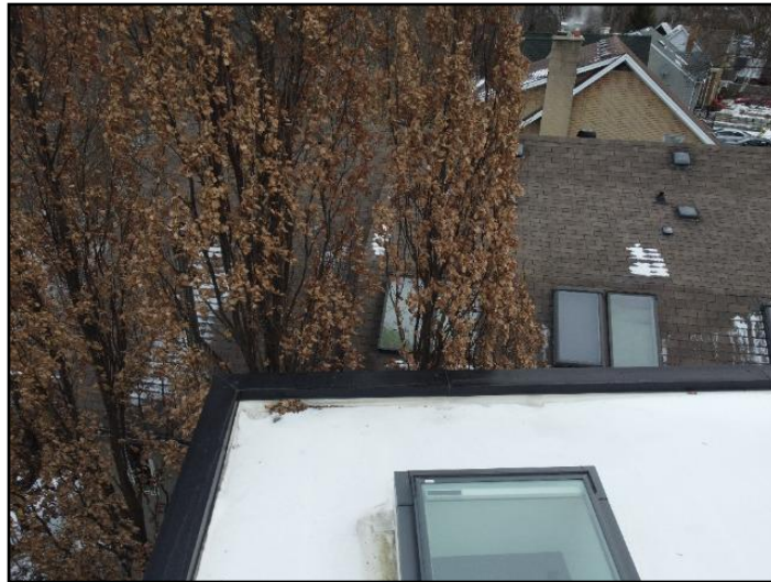
7. Trees or shrubs too close to building
