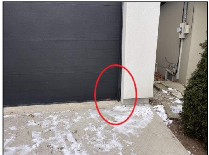
9. Weatherstripping damaged or missing.
