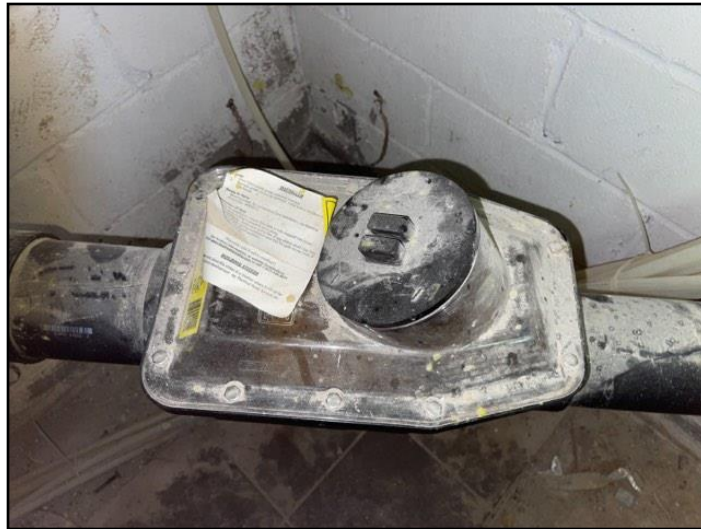
37. Present. These valves help prevent sewer...
