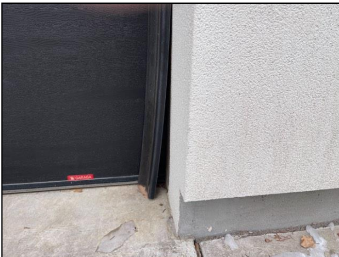
8. Weatherstripping damaged or missing.
